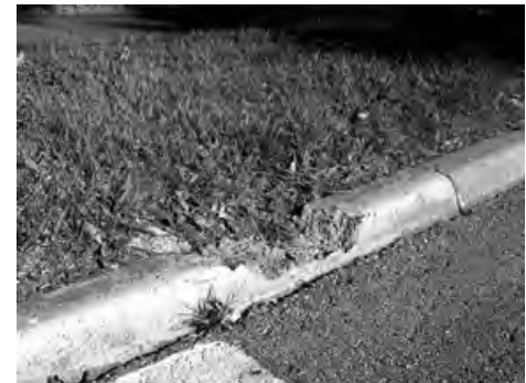
Cracked curbs are unsightly and make parking and walking difficult.
