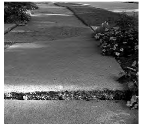
Uneven, cracked sidewalks can be dangerous for walkers, especially when combined with sweet gum balls. Not only can residents be injured, many are now walking in the street instead of on sidewalks.
