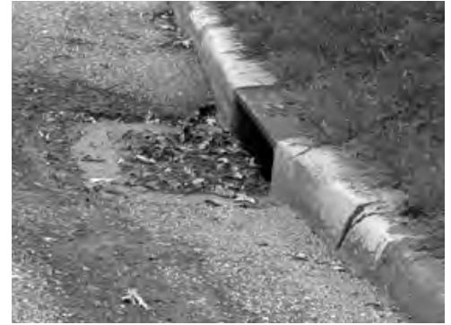
Ponding, or standing water in the gutters after a heavy rain, is troublesome for homeowners, drivers and parkers, as well as a health and safety issue.
